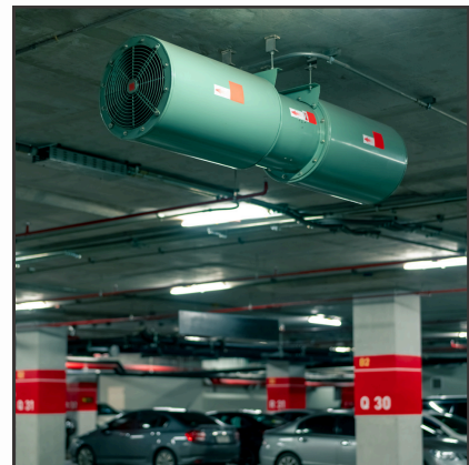
Basement Ventilation Fans
