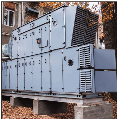
Air Handling Units
